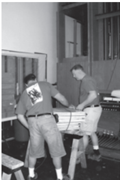
Workers from the Bedient shop remove components of the Schlicker studio organ at the University of Iowa for restoration (Photo by William Dickinson)
