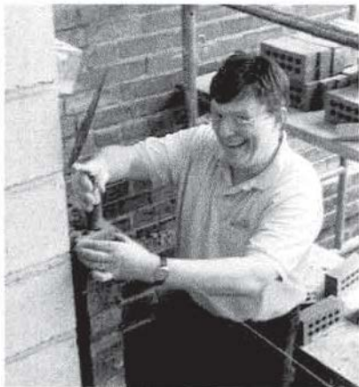
John-Paul Buzard lays brick at the entryway to the Buzard Organ Company addition, summer, 2002
