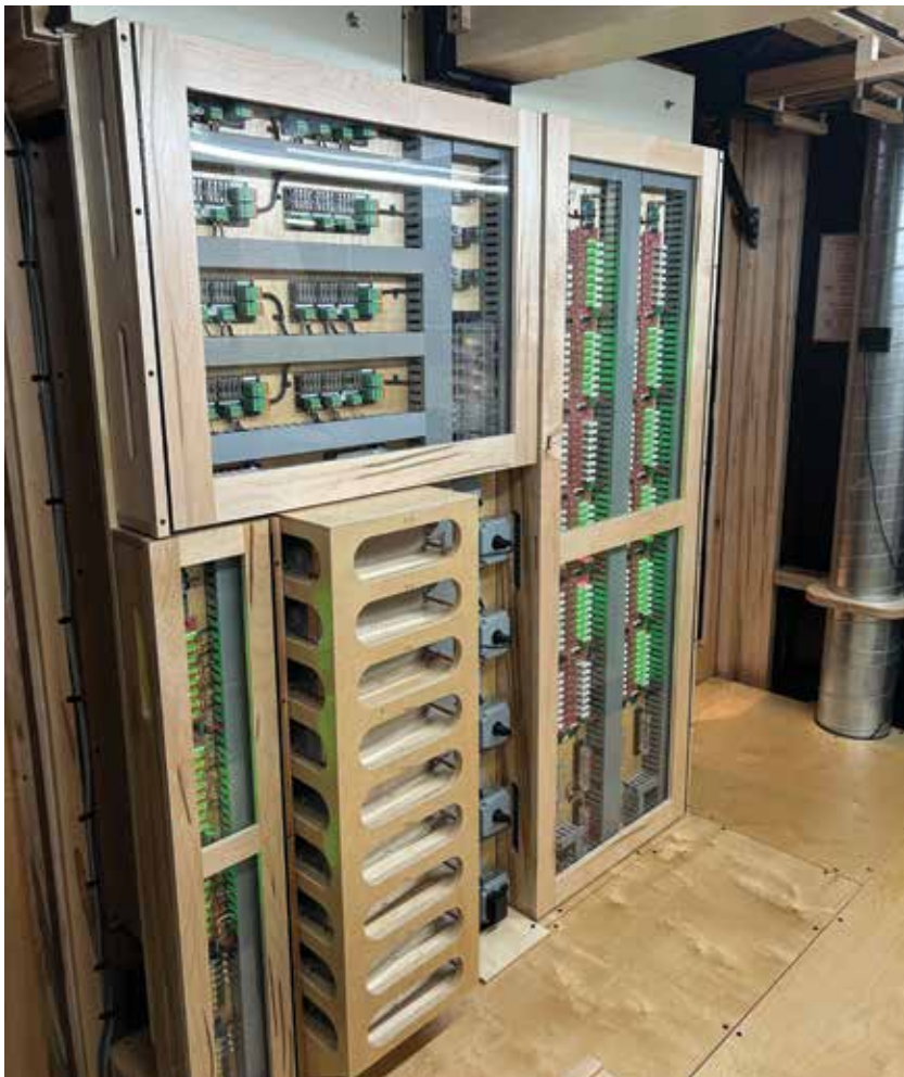
The Opus-Two ICS control system shown here with fusing blocks and low-voltage power supplies
