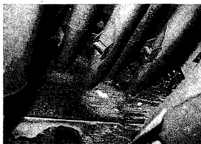
The original Wicks chest damaged beyond repair or salvage by water from a leaky roof.
