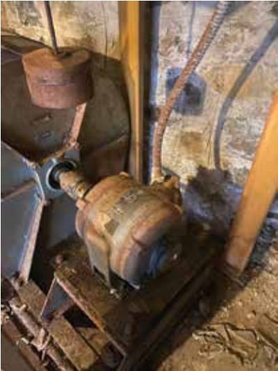
Rusty, dirty blower room (photo credit: John Bishop)
