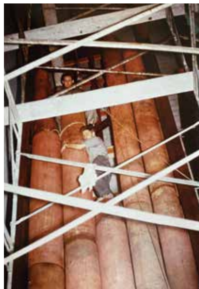
Saint Mark's Cathedral, Seattle, Washington, 1965 D. A. Flentrop organ. The Pedaal 32' Prestant copper pipes being assembled in interlocking sections
